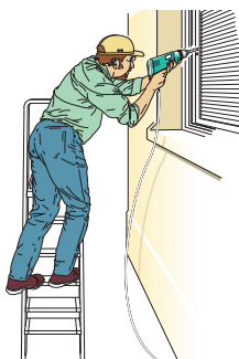
Figure 2a Incorrect - steps side-on to work activity
